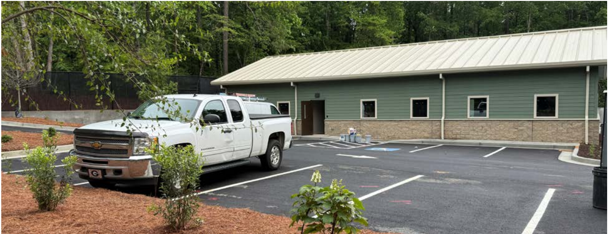
Brook Run Maintenance Facility: Steel structure and roof were completed for both buildings, with the warehouse building nearing completion.
